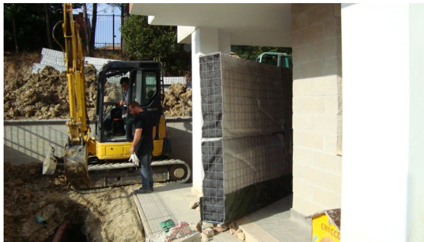
Modules DRENTER assembled in one strip waterproofed at the bottom, before laying into the trench.
